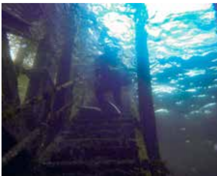
A difficult entry at Bardentarbat Pier
